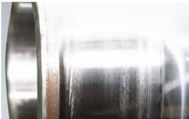
Photo 4.5 Part: Inner ring of a spherical roller bearing Symptom: Partial smearing occurs circumferentially on raceway surface Cause: Poor lubrication
